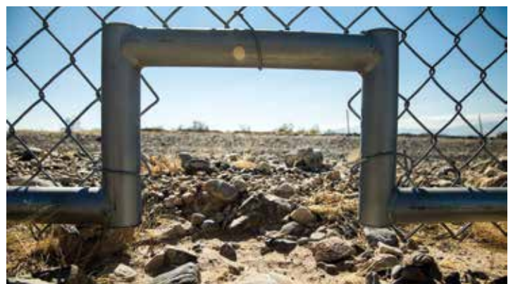
Tortoise holes in fencing
